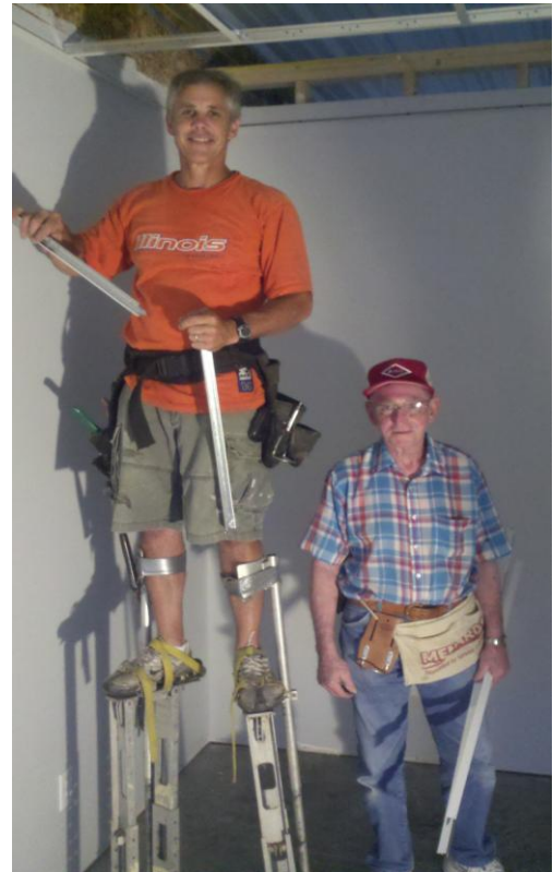
Pastor Duane and Jim Millsap work on hanging ceiling tile in the Life Center. We look forward to an early fall Open House as the building nears completion. We have been blessed with some of the most wonderful volunteer! Many thanks to you all!
